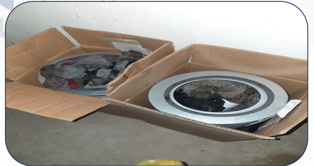
Replaced Parts During Generator Maintenance
